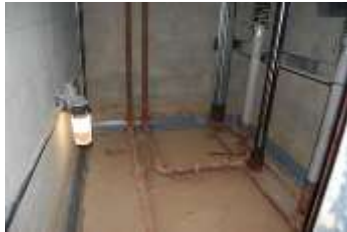
Gambar 5. Pit (Lekuk Dasar) Elevator
