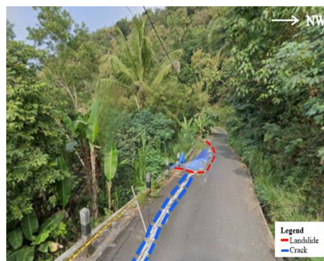
Figure 1b. Landslide Conditions
