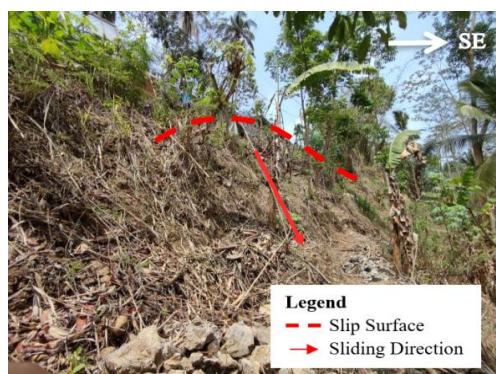
Figure 1a. Failure Pattern
