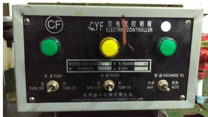
Gambar 3. Electric Controller OWS
