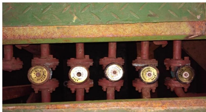
Gambar 4. Pipa Manifold line OWS
