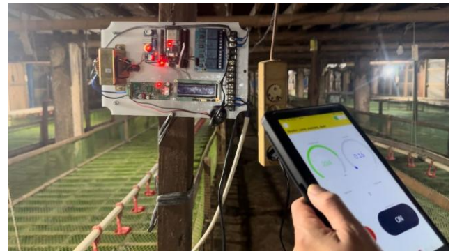
Fig 6. Testing of the IoT-based monitoring and control system in the closed poultry house at Wonolopo, Mijen
