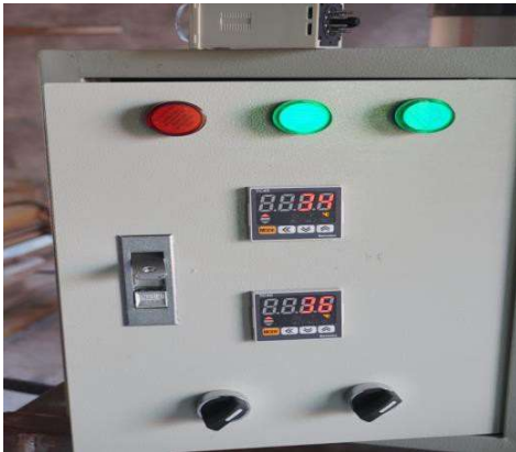
Figure 3. Design and Construction of On Off drain Dryer Control Panel (source: syahid, 2020)
