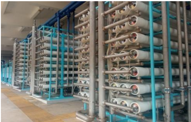
Fig 3. Reverse Osmosis at PLTU PT BAI
