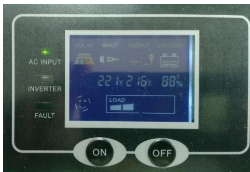
Fig.7. Battery charging indicator from solar cells
